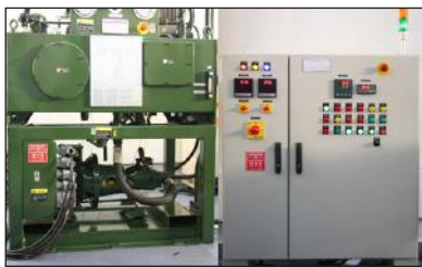
Electrical Control Panel
