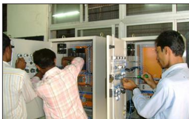
Manifold Block Control System
